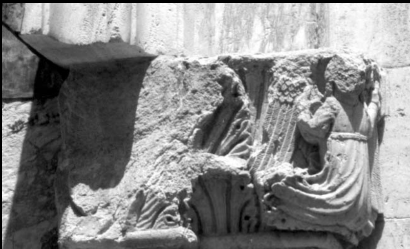
The façade of the church, capital with the representation of an angel, typical damages of the stone
