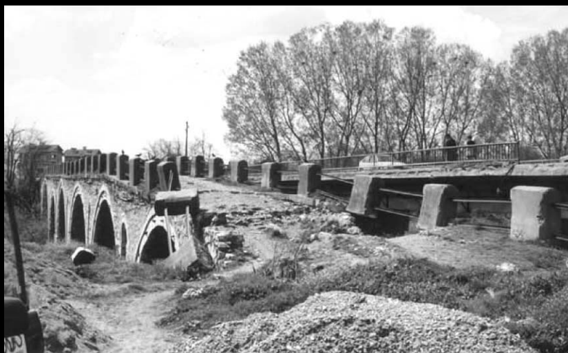
The damages of the cobble pavement on the bridge
