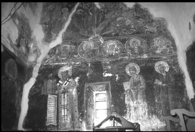
The south wall of the nave, donor's portrait and typical damages of the frescoes
