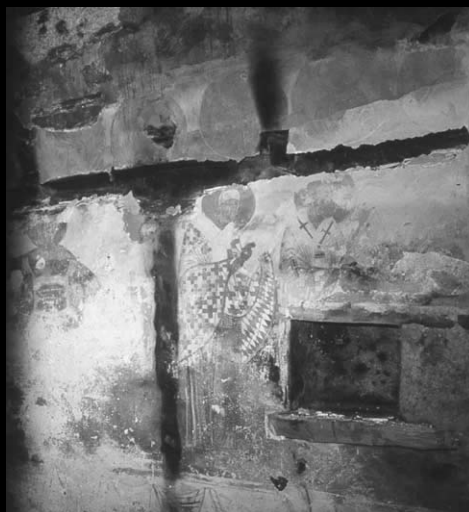
The south wall of the nave, frescoes after the fire and burned wooden beams in the wall
