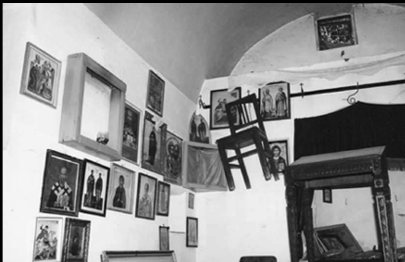
The interior after the deterioration
